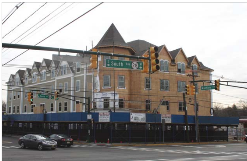
Benjamin B. Corbin for The Scotch Plains-Fanwood Times WORK IN PROGRESS...Fanwood Crossing, the multi-use development on the corner of South and Martine Avenue, will be complete by early summer. Fanwood Mayor Colleen Mahr said retail tenants that fit the needs of the community are being sought.
