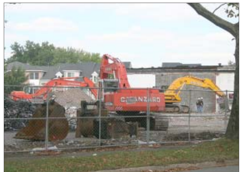
Benjamin B. Corbin for The Scotch Plains-Fanwood Times CLEANING UP SHOP...Workers demolish a building that formerly housed La Belle Cleaners and The Mattress Factory on North Avenue in Garwood as part of a new redevelopment project.
