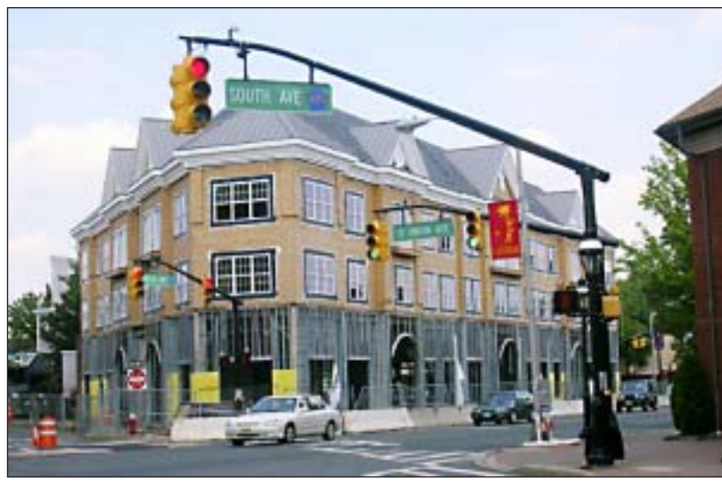
MAKING AN APPEARANCE...The Cranford Crossing development in downtown Cranford forges ahead and is taking shape for its coming role in the business district. See www.goleader.com/photos.
