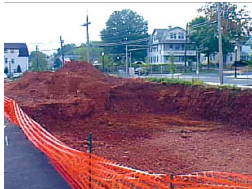
THE BIG DIG...Work has resumed at the apartments on the corner of Central Avenue and Cacciola Place in Westfield.
