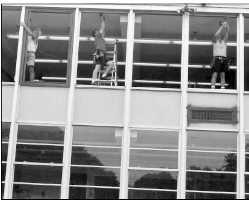
IMPROVEMENTS UNDERWAY... Signs of improvement at Westfield High School are already visible as crews work to install new windows this summer. The new school bond referendum, passed by Westfield voters in December 2000, will fund major improvements and an addition to the building, which will be 50-years-old this year.
