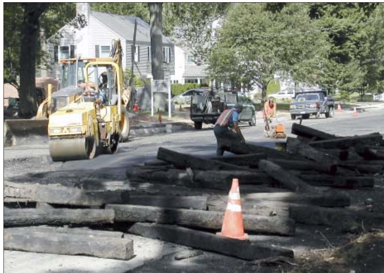
THE BIG DIG...The northern end of Elm Street in Westfield gets completely rebuilt as part of the town's program to permanently repair the street. Old rail ties and Trolley tracks, which were buried beneath the surface for decades, are removed.
