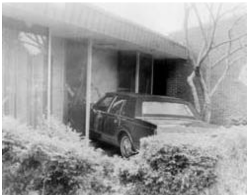
Car Damages Library Wall
