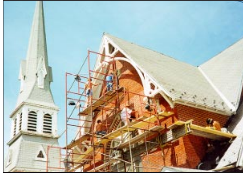
GETTING A FACE LIFT... The outside of the sanctuary of Scotch Plains Baptist Church, which dates back to 1870-1871, is currently under construction at a cost of approximately $29,606. Pictured on the scaffolding are workers of Statewide Restoration Inc., which has been contracted for the cleaning and brickwork. The general contractor for the project is Skinner and Cook Inc. of Roselle Park.
