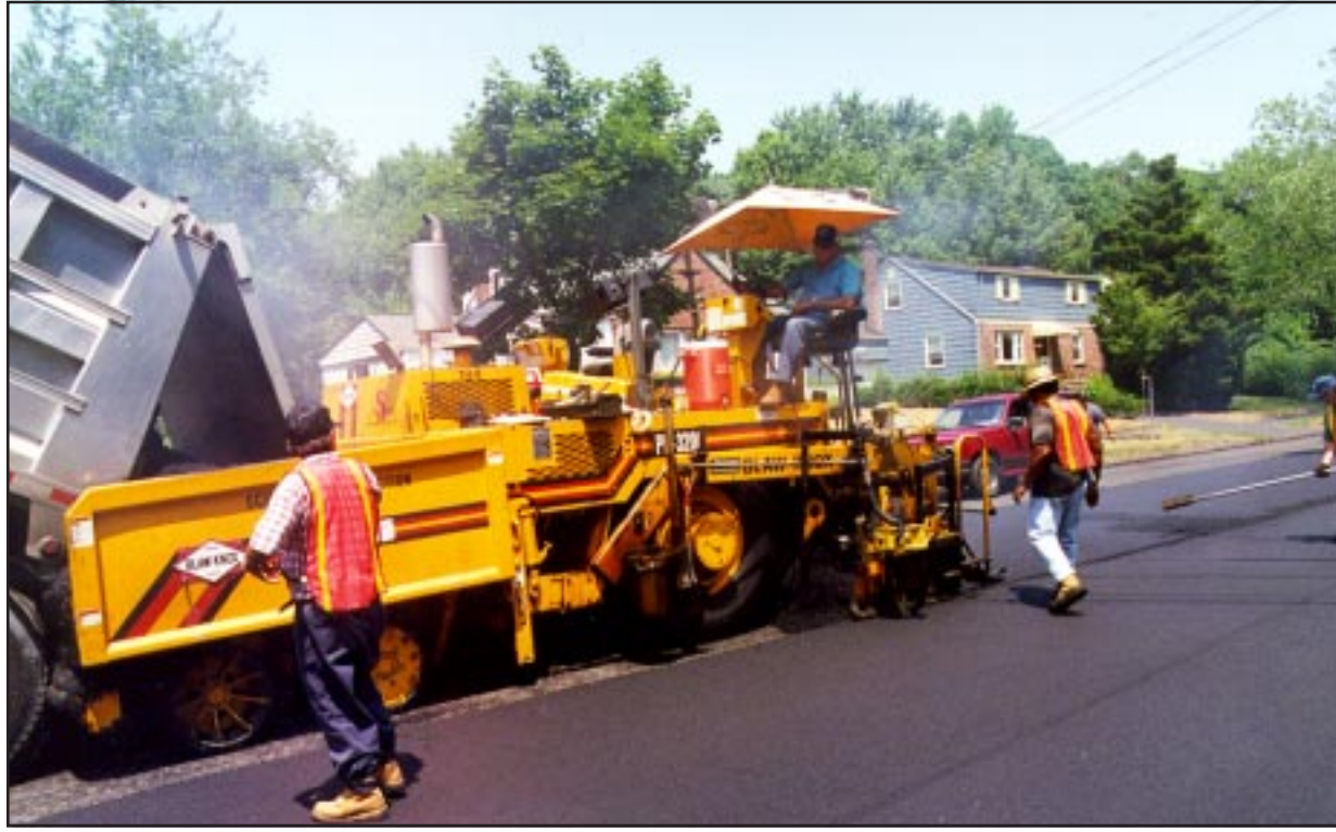
FRESHLY PAVED...Workers are shown last week paving Midway Avenue, the extension of North Avenue, in Fanwood. The work on North and Midway created traffic havoc while the paving work was completed. Paving and other roadway work will continue through the fall on both Union County and town roadways.
