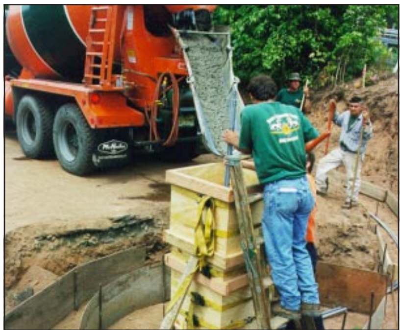
LAYING THE FOUNDATION...Public Works employees prepare the foundation last Thursday for Fanwood’s Millennium Clock, which will be unveiled during the borough’s annual Fanny Wood Day festival on Sunday, September 26, in the downtown. The clock, paid for through Fanny Wood Day revenues along with contributions, will stand near the Fanwood Train Station at South and Martine Avenues.
