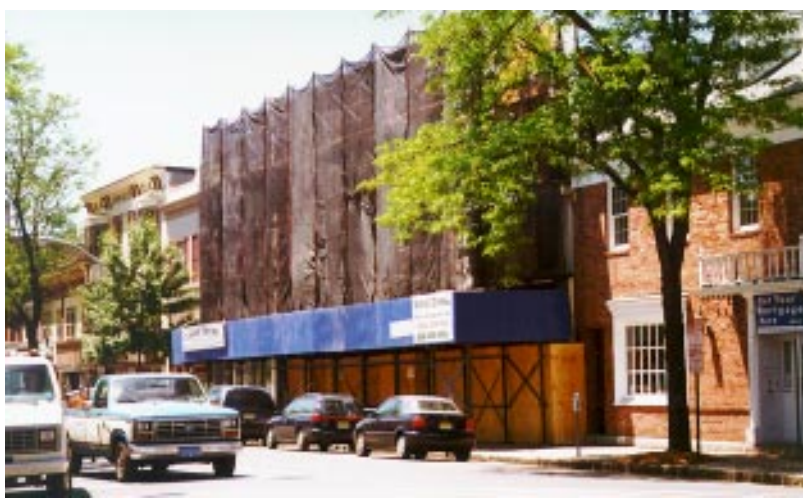
GETTING A FACELIFT... Renovation work has begun on buildings located at 159-169 East Broad Street. Apartments on the second and third floors are being completely renovated. Classic Thyme will be joined on the ground floor by Nine West in the old Epstein Bootery space, while Ann Taylor will be moving into space previously filled by Milady's and Village Curtains.
