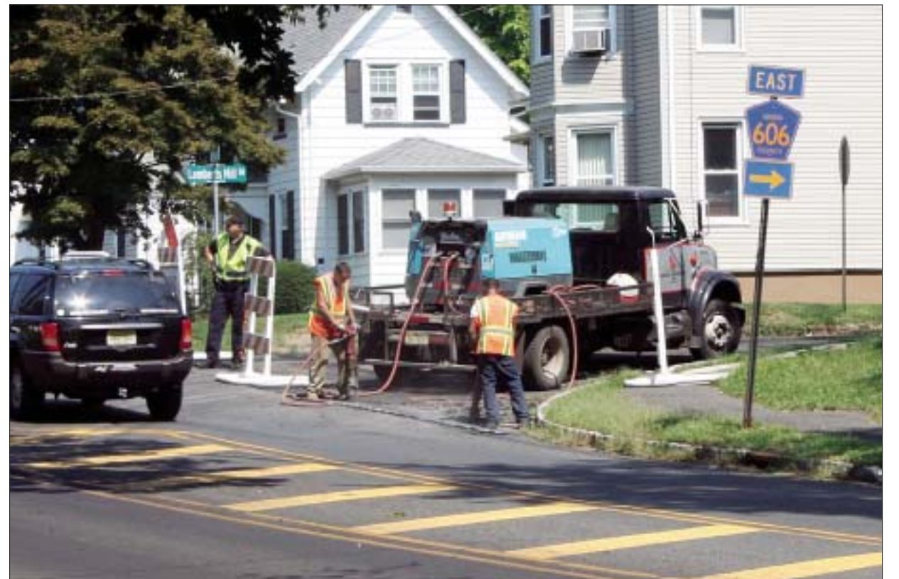
Benjamin B. Corbin for The Scotch Plains-Fanwood Times MEN WORKING... Contractors for the County of Union work at a fast pace to resurface many of the county roads prior to Labor Day. Pictured above, the men are working this week on Lamberts Mill Road in Scotch Plains.
