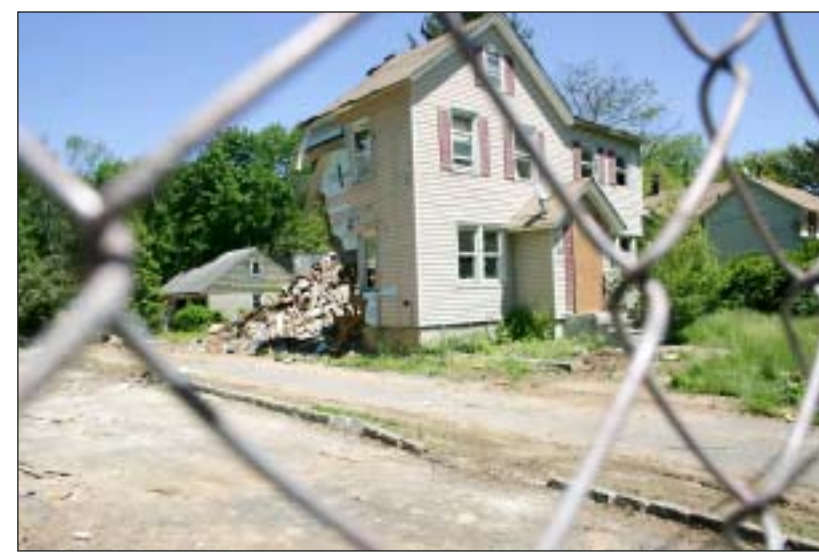
Fred Rossi for The Westfield Leader STATE OF REPAIR... Two Prospect Street properties owned by Alan Chrono, including one pictured above, are being demolished after a nearly two-year delay. The properties have been cited for property-maintenance-code violations and housed S.W.A.T. training during the time. Neighbors have continued to complain at Westfield Town Council meetings about the dilapidated states of the two homes. Once demolished, Ralph Rapuano, Jr. will develop three new homes. According to town policy, a house going through the subdivision-approval process cannot be demolished before receiving the authorization of the town.
