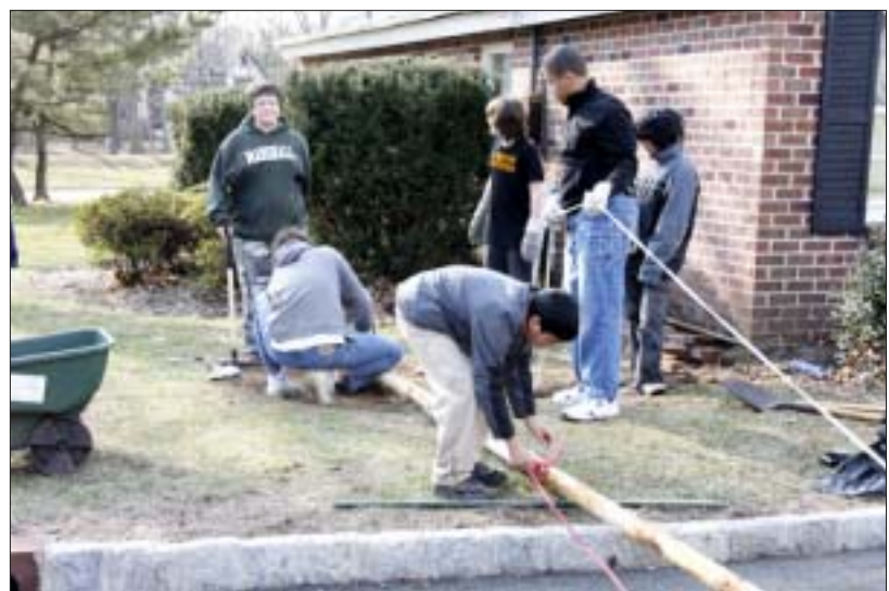
HEALTHY MEETING...The Fanwood Rescue Squad's corroded, 30-year-old flagpole is being replaced this week by Scouts of Troop 104, led by Eagle Scout candidate Courtney Slaten, who is also a member of the squad. Pictured is the old flagpole after it was removed last weekend. The new pole will stand a few feet away, surrounded by new pavers.
