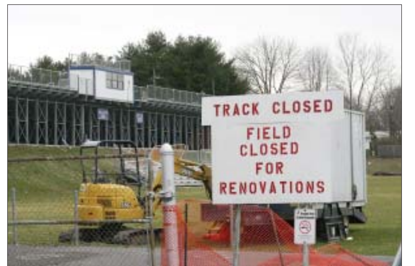
NOT RUNNING...The Scotch Plains-Fanwood High School field is closed awaiting construction of the turf field addition. Neighboring towns of Plainfield, Kenilworth and Cranford are helping by providing facilities for the track team to practice.
