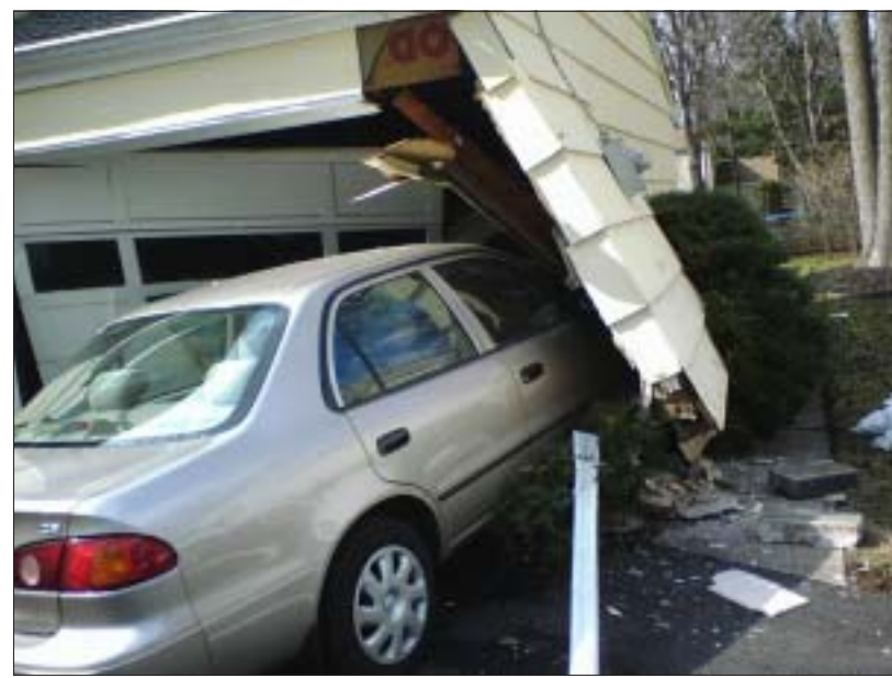
OOPS... Last Saturday afternoon around 1 p.m., a Westfield woman at 115 Roger Avenue errantly drove her vehicle into her garage, causing extensive damage.
