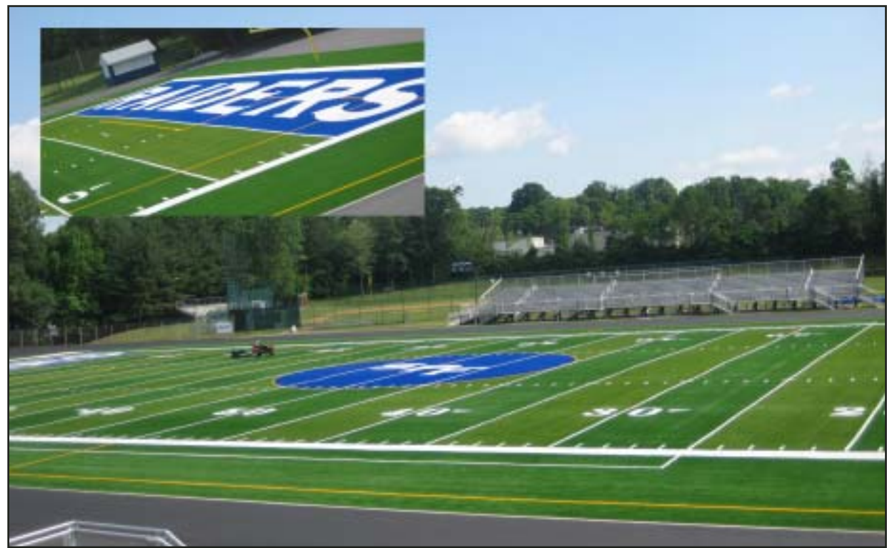
READY FOR GRADUATION...With the turf project almost complete, the new Scotch Plains-Fanwood fields are in great shape for this year's graduation ceremony. Work on the track will begin after graduation.
