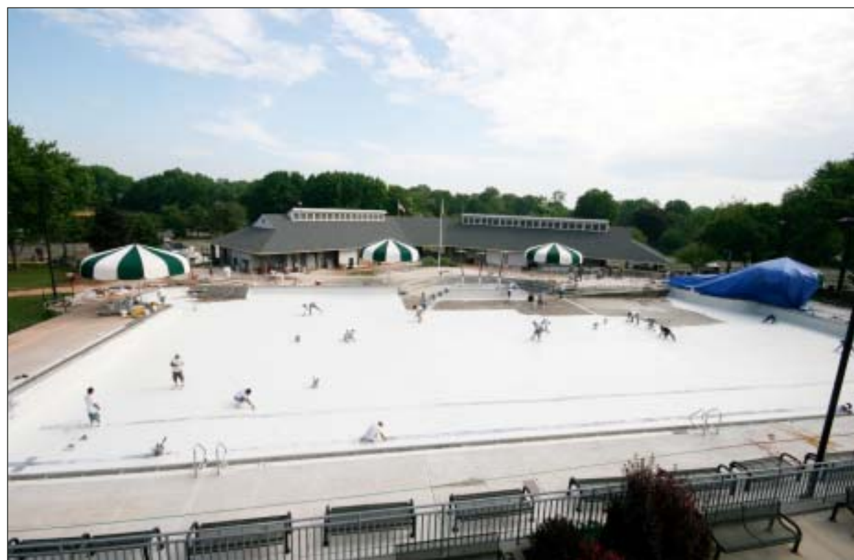
Greg Ryan for The Westfield Leader READY FOR THE HEAT WAVE...Last weekend, workers put the final touches on the Westfield Memorial Pool Complex before filling it with water. After a one-week postponement, the pool is being given finishing touches to be ready for the Saturday, June 14, opening. Extreme weather conditions were said to have caused the opening date to be pushed back. See pool photographs at goleader.com/photos.
