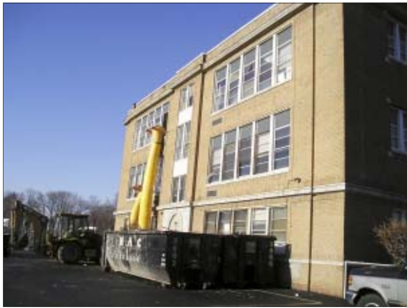
CHUTES AND LADDERS... Not a giant water slide, the early childhood center at Westfield's Lincoln School undergoes extensive interior demolition and construction debris disposal last week.
