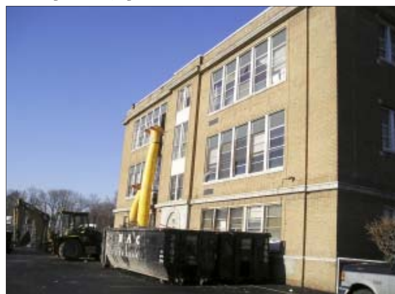
CHUTES AND LADDERS... The early-childhood center at Westfield's Lincoln School undergoes interior demolition and construction debris disposal last week. The chute is placed for safety reasons, according to Westfield Public Schools Business Administrator Robert Berman. Instead of dropping debris from three stories high, with the chance of particles landing in the surrounding neighborhood, the chute forms a protective enclosure for the passage of demolition materials into the dumpsters.
