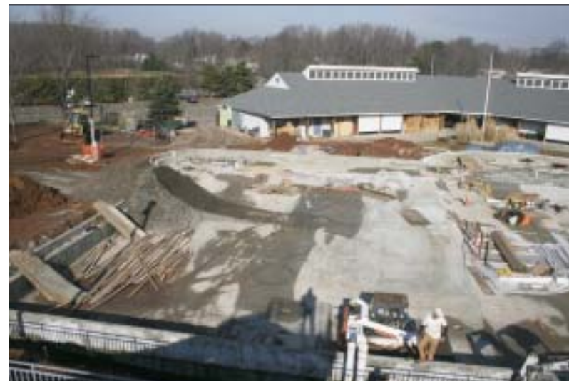
POOLING TOGETHER...The Westfield Memorial Pool complex undergoes reconstruction to meet its spring deadline for reopening. Westfield Recreation Director Bruce Kaufmann reported that the work is on schedule.
