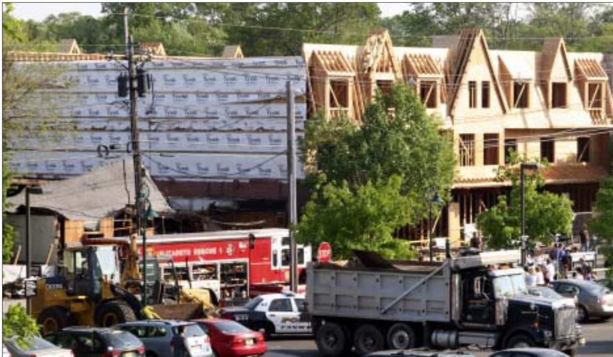
COLLAPSE (May 17) ...The collapse of a concrete firewall at the South Avenue Station Mews redevelopment project brought down the roof of Livingston-Wilbor Corporation, left, on May 15. The collapse trapped three individuals inside the business. Two injured people were Medivac'd to Robert Wood University Hospital in New Brunswick. FULLY ENGULFED (January 25)...A fire broke out in Charlie Brown's restaurant located on North Avenue around 4 a.m. on January 24. The Scotch Plains Fire Department responded along with mutual-aid units from surrounding towns. The restaurant burned to the ground.
