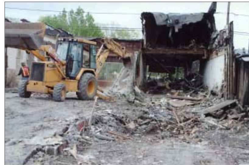
REDEVELOPMENT BEGINS (May 11)...Work begins on the first project of Fanwood's Downtown Redevelopment. Plans call for the demolition of two buildings at Second and South Avenues. The buildings were previously occupied by M.I.P. Printing and the Brass Works. Sanguiliano Enterprises is conducting the demolition and recycling the concrete, metal and wood. Ron Marcovechio, proprietor of the Fanwood Clipper, is developing the property, which will feature first-floor retail space and two floors of apartments.
