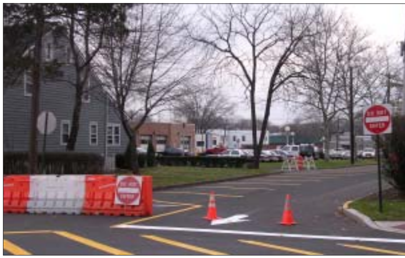
Fred Rossi for The Scotch Plains-Fanwood Times CLOSED TO TRAFFIC...Senger Place behind the Scotch Plains Police Department has been closed to traffic during construction at the Scotch Plains Municipal Building on Park Avenue.
