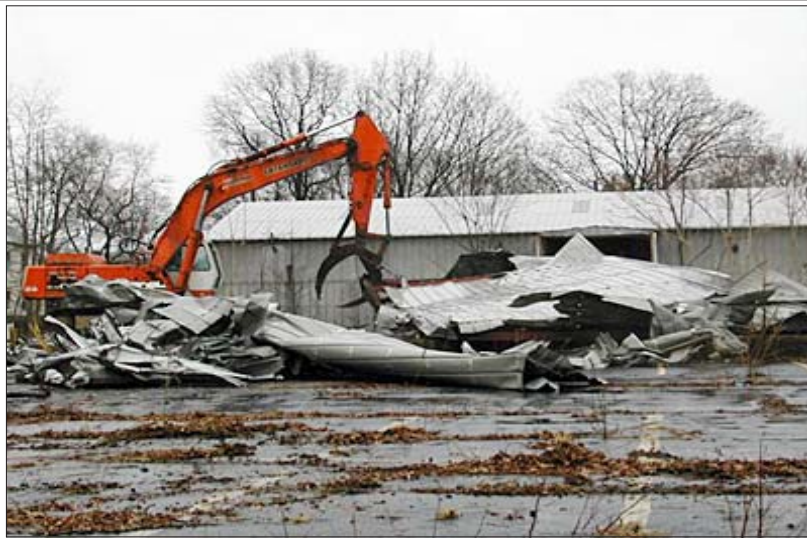
OUT WITH THE OLD...The old Thomas and Betts building, located across the street from the Garwood ShopRite, was demolished last week to make room for 21,000 square feet of residential and commercial development in a Main Street-like setting. The project is expected to be completed by the fall.
