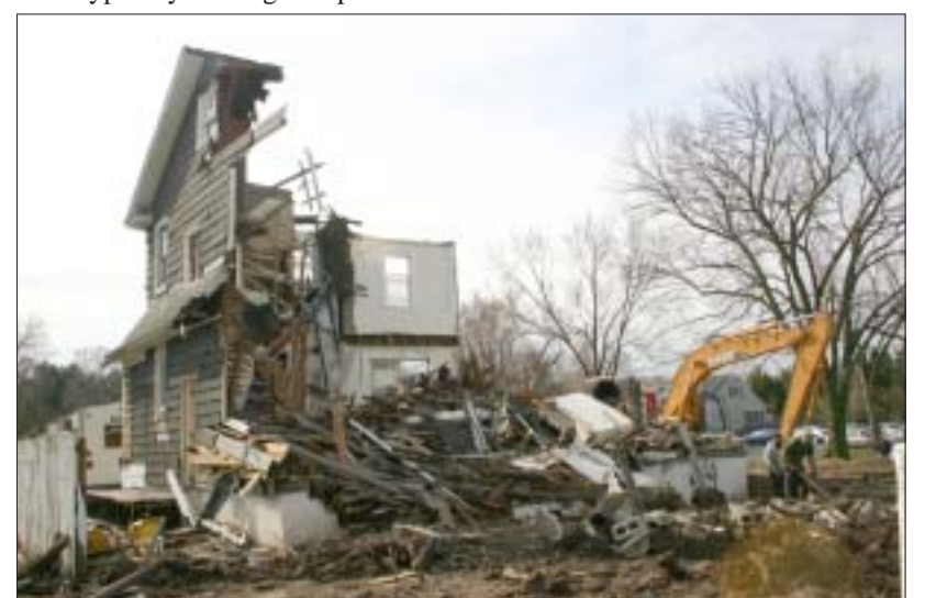
NEW CONSTRUCTION...Messercola Brothers Builders Co. is demolishing a house to make way for new construction on South Avenue in Fanwood.
