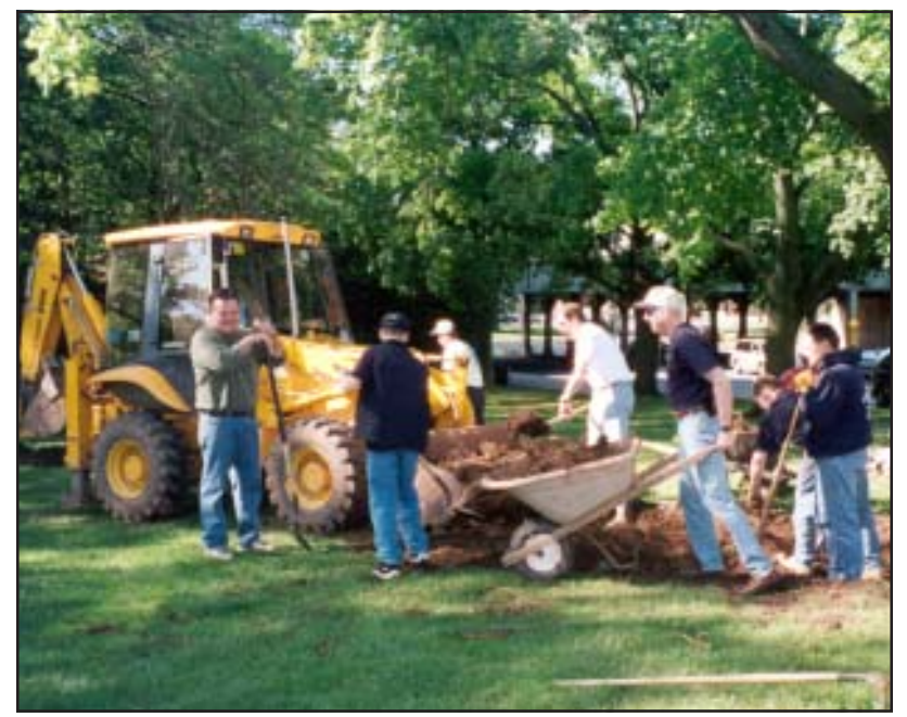
DIGGING IN...Construction began on Saturday, May 11, on the site designated for the September 11th Memorial Park on the corner of East Broad Street and North Avenue in Westfield. Under the direction of Craig Stock, landscape designer for the project, volunteers from the Jaycees and the Friends of Dean Eberling began initial excavation of the area that will house a glass and granite memorial honoring the victims of the September 11th tragedy.
